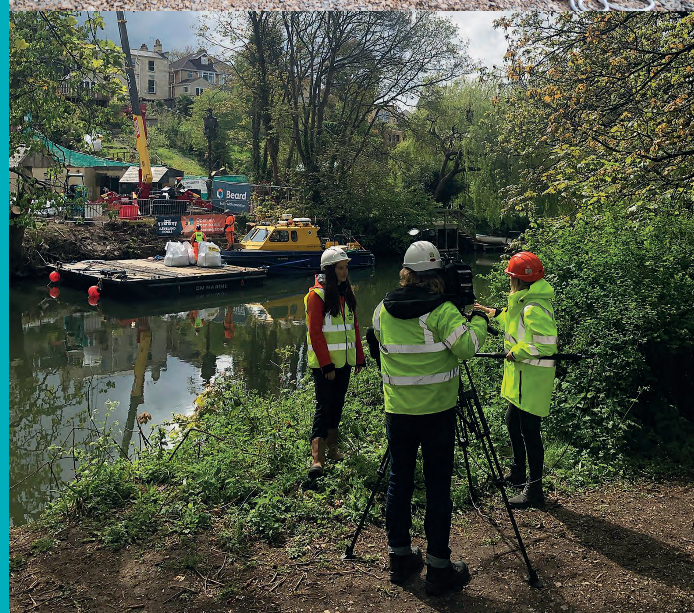
Restoration work starts. Contractors transport materials to site on a river barge, 2021.
