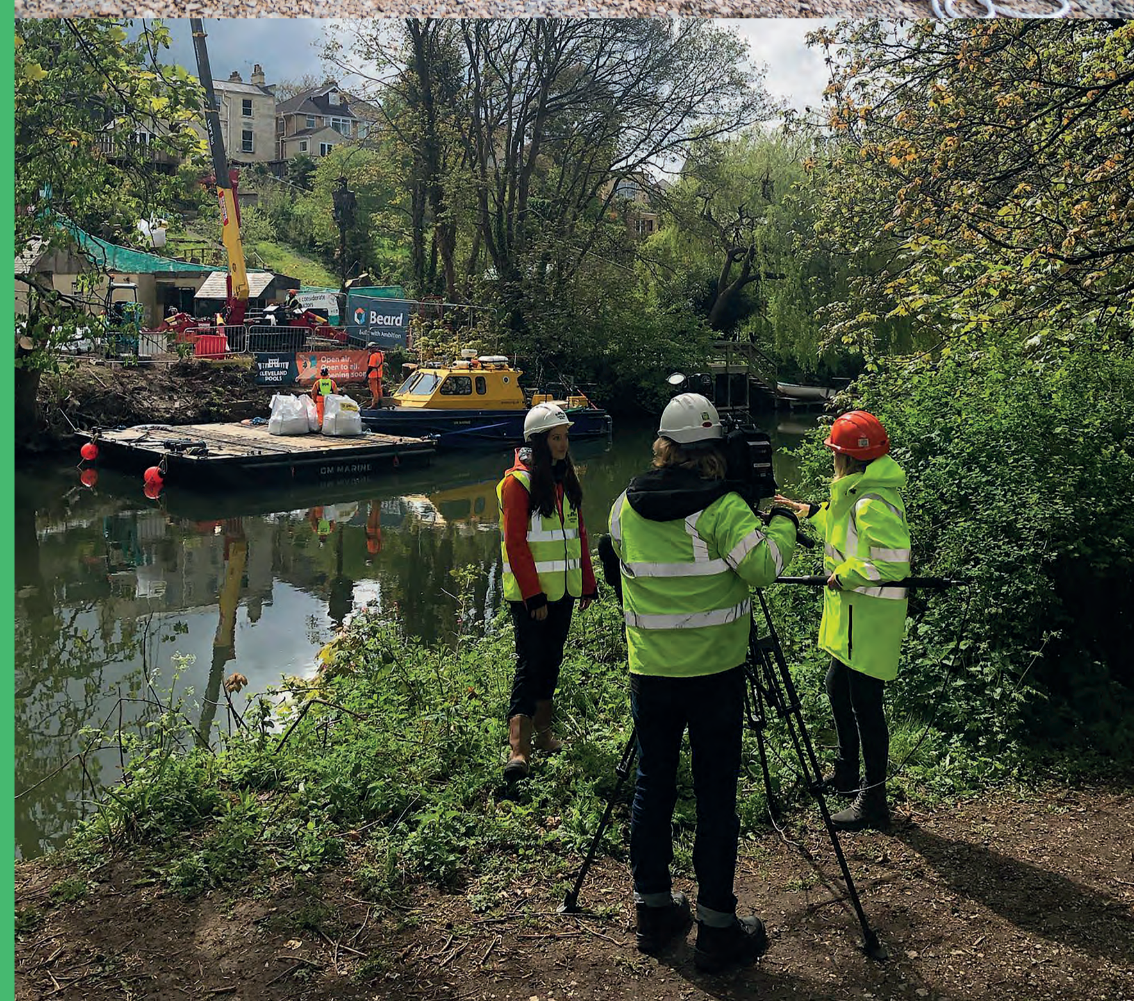
Restoration work starts. Contractors transport materials to site on a river barge, 2021.
